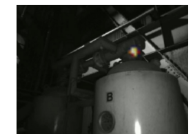
Chemical storage tank maintenance (Gas leakage)
