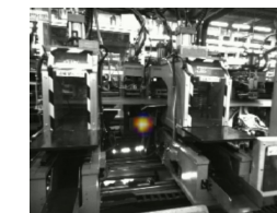
In-line facility maintenance (Compressed air leakage)
