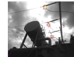
Power lines partial discharge
