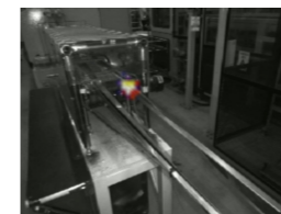
In-line facility maintenance (Compressed air leakage)
