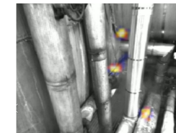
Multiple leaks in pipelines
