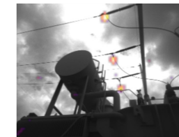
Power lines partial discharge
