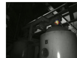
Chemical storage tank maintenance (Gas leakage)
